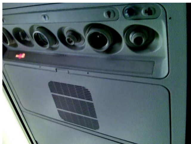
Figure 2 Personal service unit (PSU) with three gaspers, three reading lights and oxygen masks (not showing) in a narrow body cabin.
